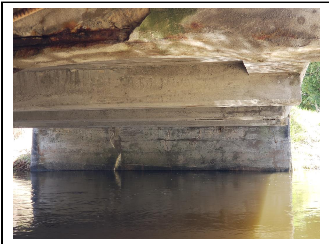
Photo 14 Moderate erosion and scaling were noted at and below the waterline on north abutment wall
