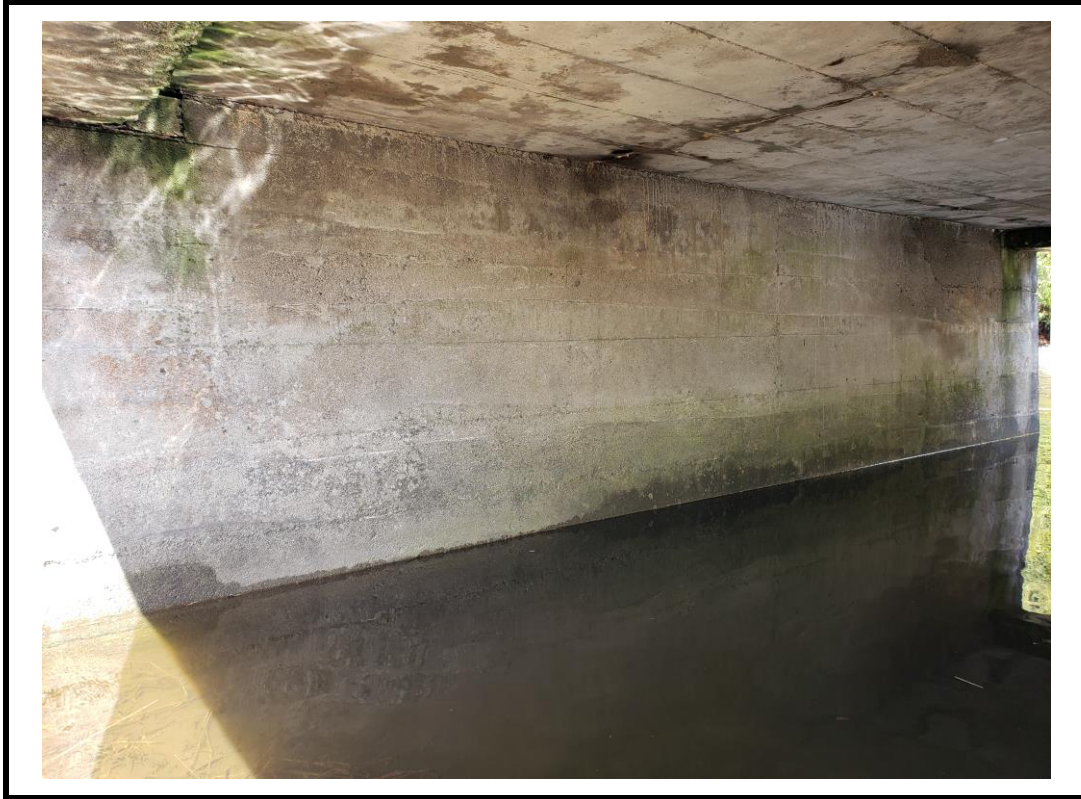
Photo 15 Moderate erosion and scaling were noted at and below the waterline on south abutment wall
