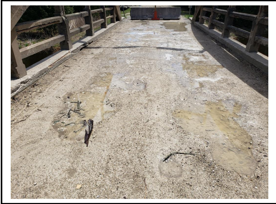
Photo 9 Spalls in exposed concrete deck top
