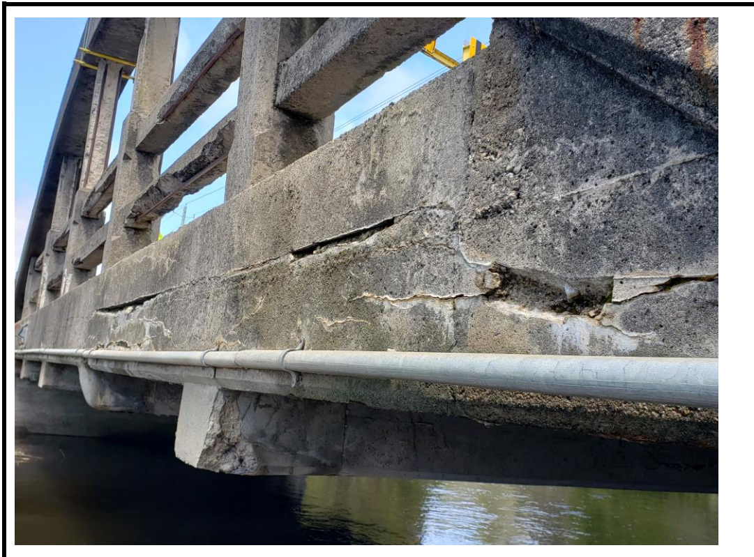
Photo 16 Wide cracks noted at underside of west chord near south end
