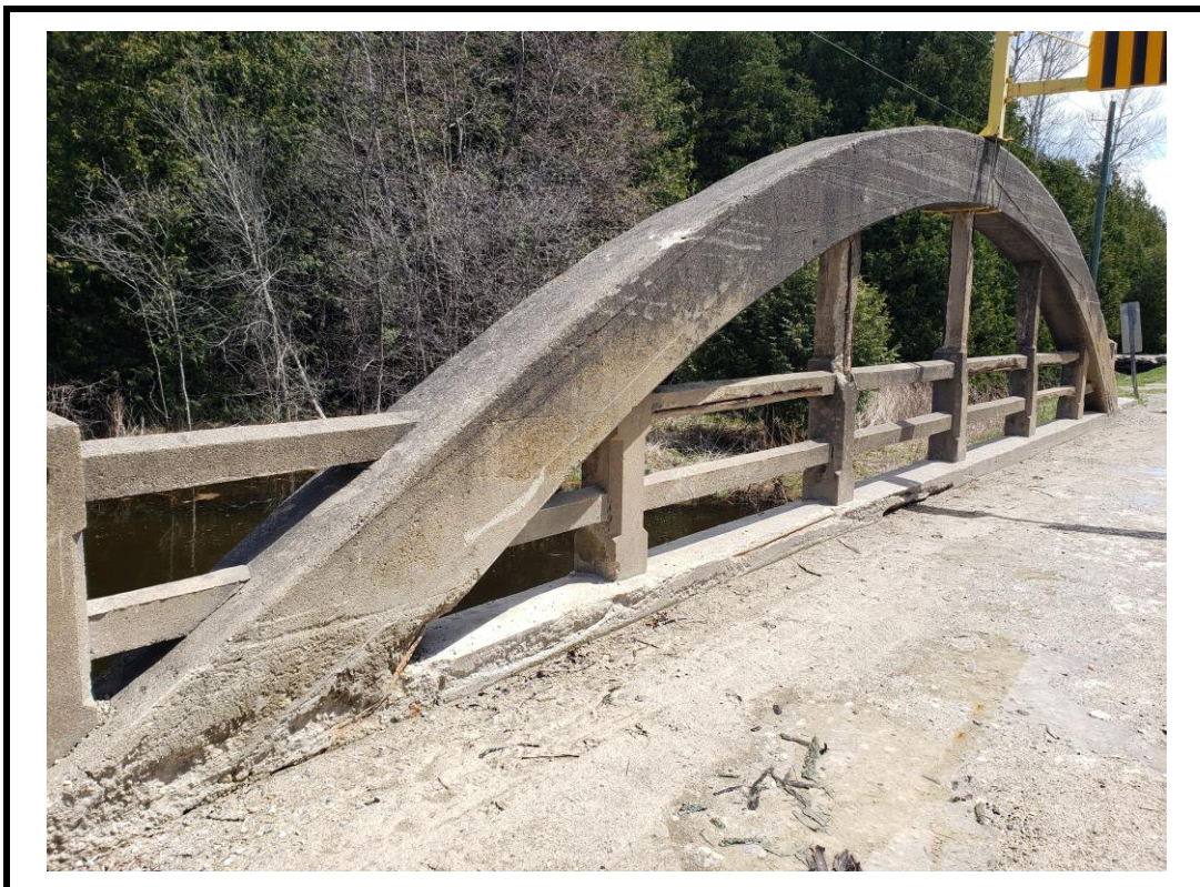
Photo 8 Severe spalling with exposed corroded rebar at rail in deck barrier
