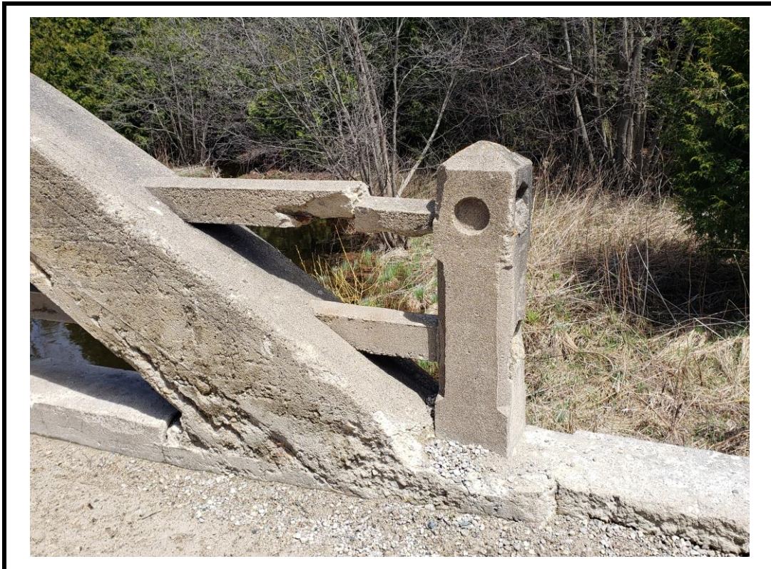
Photo 10 Spall with exposed corroded rebar and sheared railing in deck barrier at southeast corner
