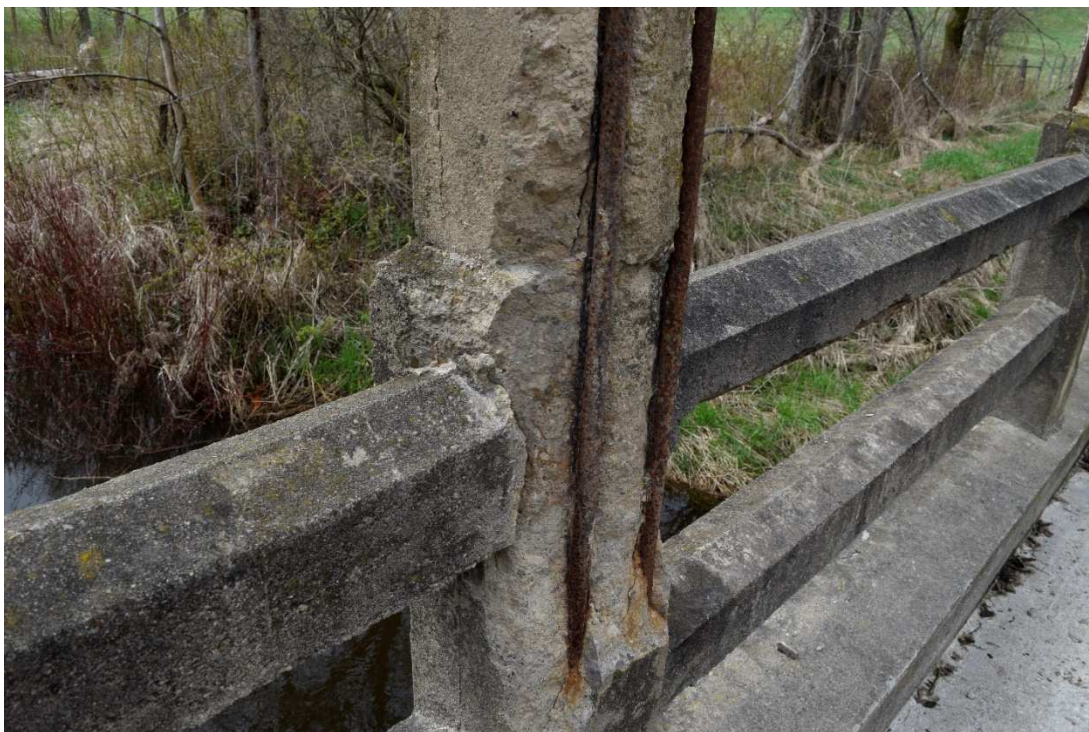
FIGURE 7: BRIDGE 3-E, TYPICAL EXAMPLE OF DETERIORATION, EXAMPLE IS OF SUPERSTRUCTURE CENTRAL SUPPORT
