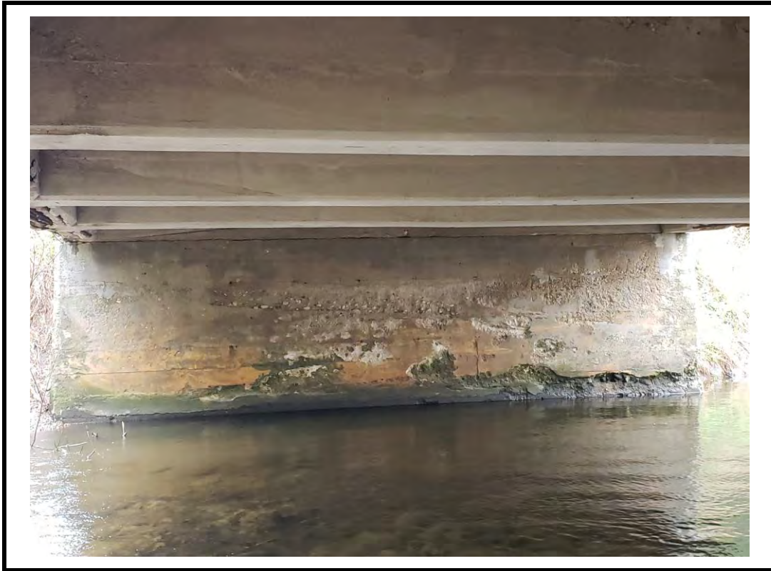
Photo 13 Severe spalls with concrete disintegration noted on south abutment wall
