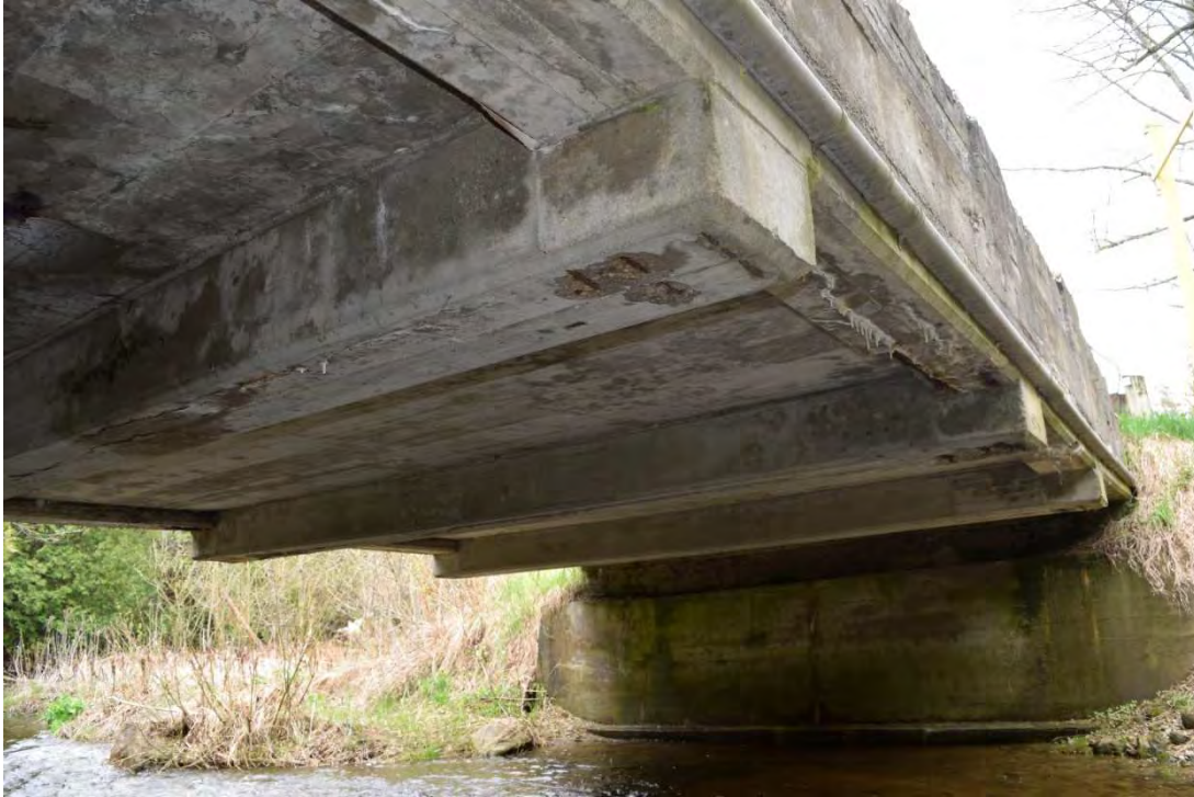
FIGURE 29: BRIDGE 7-E, EVIDENCE OF PAST RECONDITIONING OF THE BRIDGE, WHICH IS SHOWING SIGNS OF DEGRADATION
