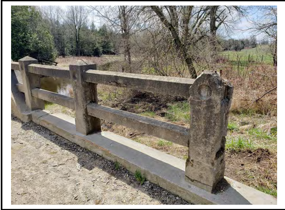
Photo 7 Concrete disintegration with exposed corroded rebar at northwest of deck barrier post
