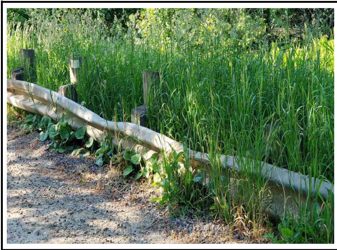
Photo 7 Collision damage noted at west approach barrier
