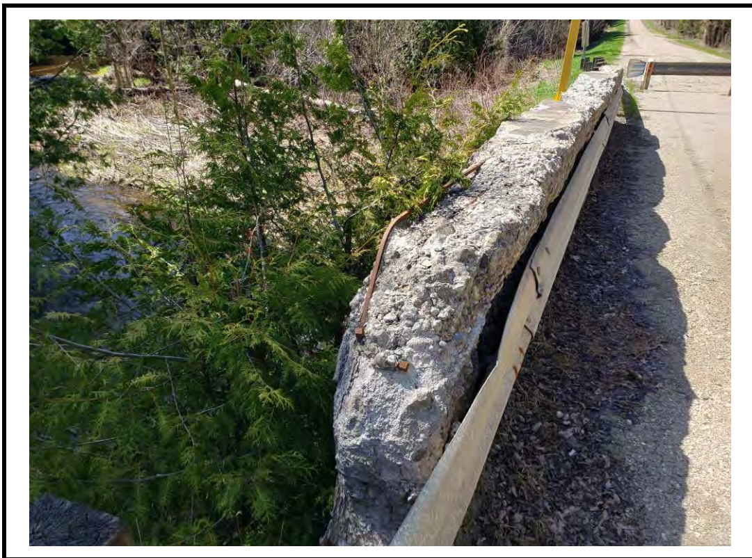
Photo 8 Traffic Barrier Disintegration with exposed corroded reinforcing
