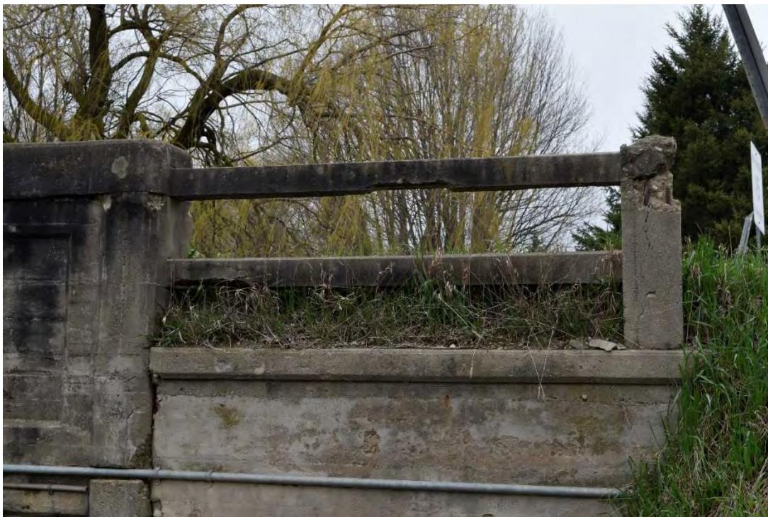
FIGURE 6: BRIDGE 2-WG, CLOSE UP OF TYPICAL GUARD RAIL DEGRADATION
