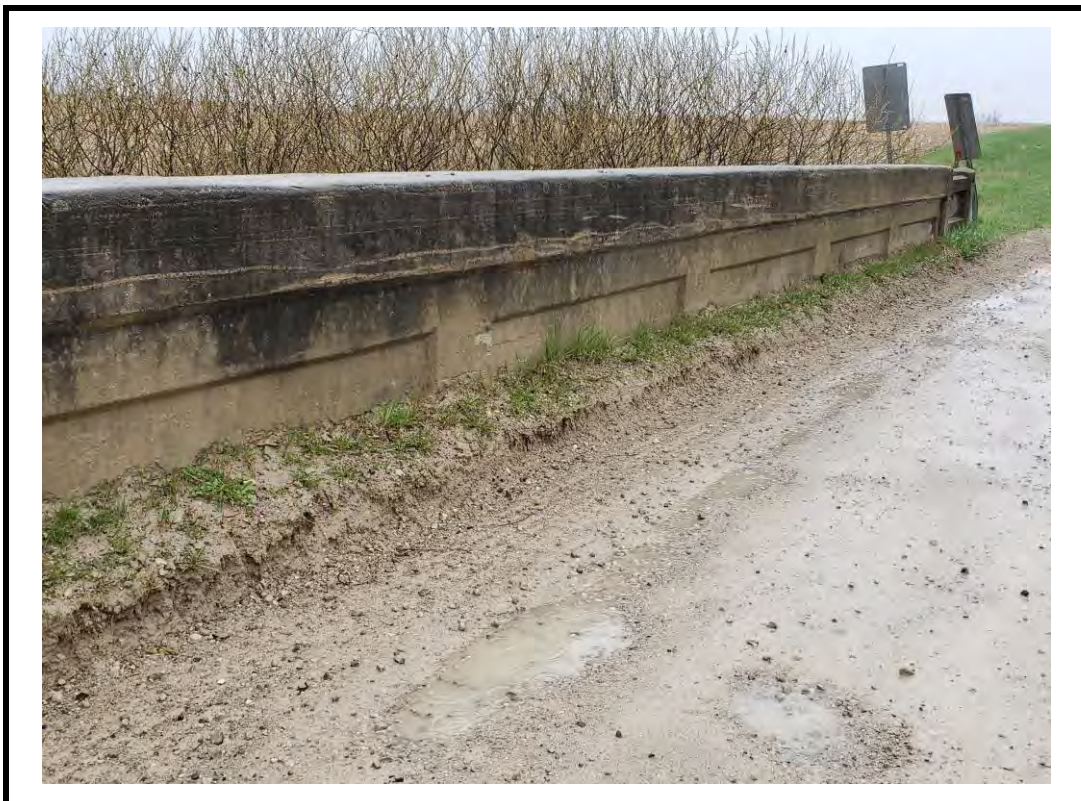
Photo 8 Disintegration with small spalls noted on east parapet wall
