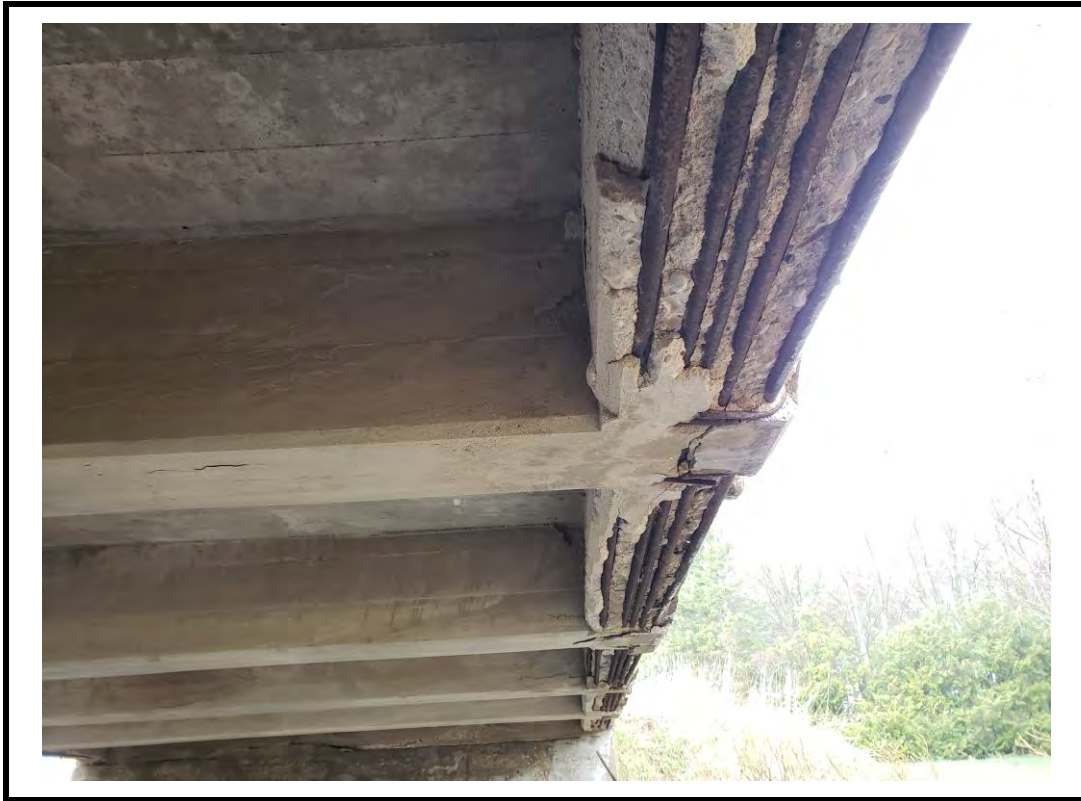
Photo 15 Sever spalling with exposed corroded reinforcement noted over the full length of west exterior beams
