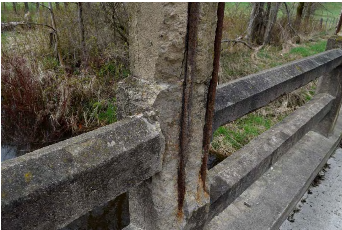
FIGURE 16: BRIDGE 3-E, TYPICAL EXAMPLE OF DETERIORATION, EXAMPLE IS OF SUPERSTRUCTURE CENTRAL SUPPORT
