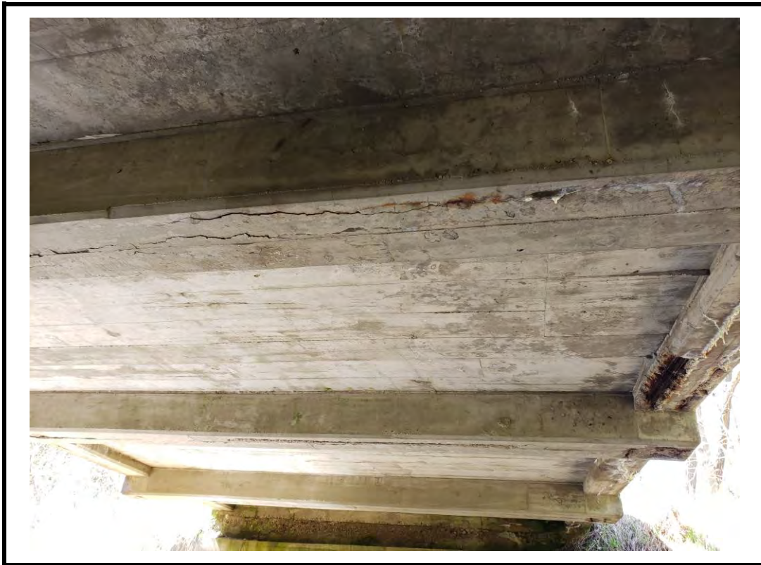
Photo 9 Delamination and spalls with exposed corroded reinforcing on soffit
