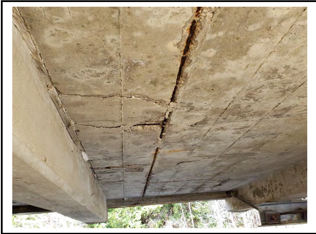
Photo 13 Large spalls with exposed corroded rebar noted at soffit in between girders
