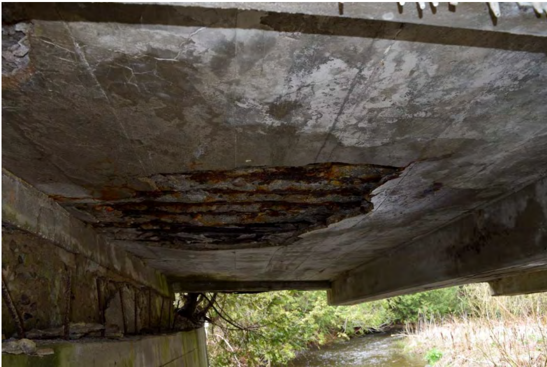
FIGURE 28: BRIDGE 7-E, EXAMPLE OF THE UNDERSIDE OF STRUCTURE, SHOWING EXPOSED AND UNSUPPORTED REBAR IN BOTH THE BRIDGE DECK AND THE ABUTMENT WALL
