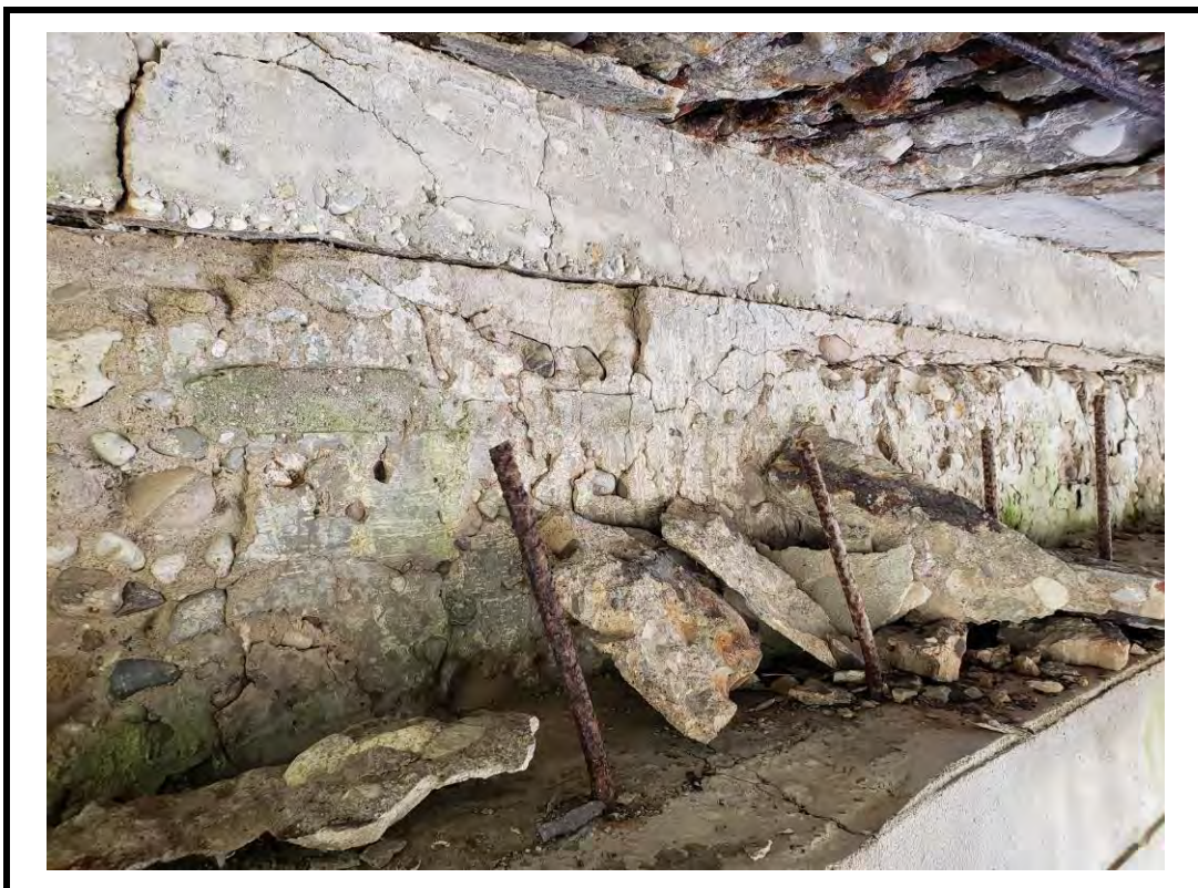
Photo 12 Exposed corroded reinforcement with severe scaling noted at ballast wall
