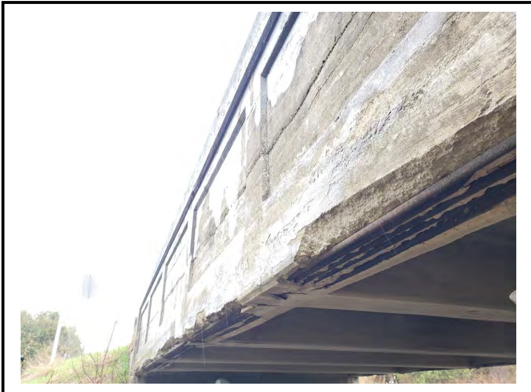
Photo 10 Severe scaling, damp stains and spalls with exposed corroded reinforcement noted on exterior parapet wall
