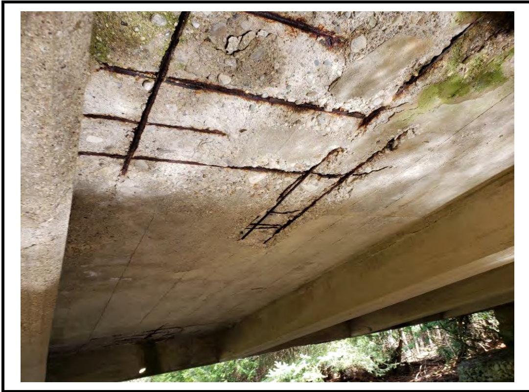
Photo 11 Spalling with exposed corroded rebar at soffit
