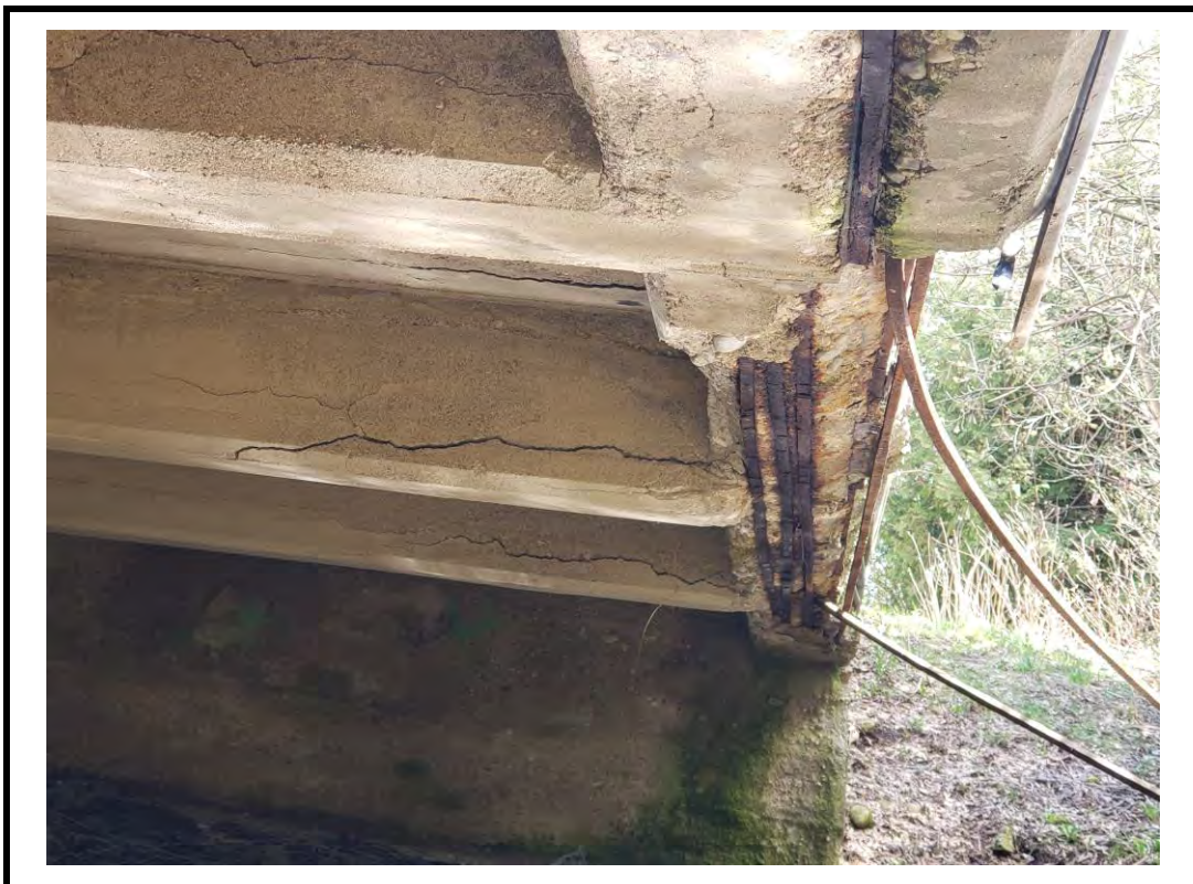
Photo 10 Severe spalling with exposed corroded rebar at underside of girder
