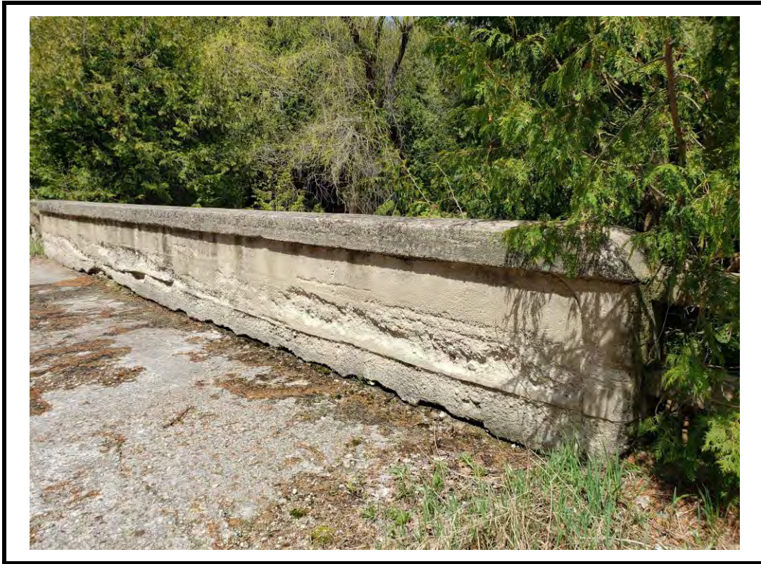
Photo 7 Severe concrete deterioration at base of deck barrier
