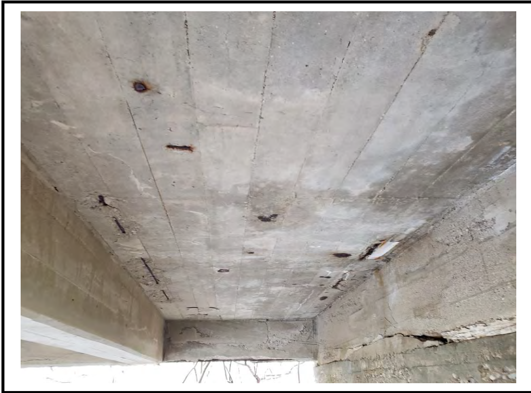
Photo 11 Medium horizontal cracks with delamination with exposed corroded reinforcement noted at soffit
