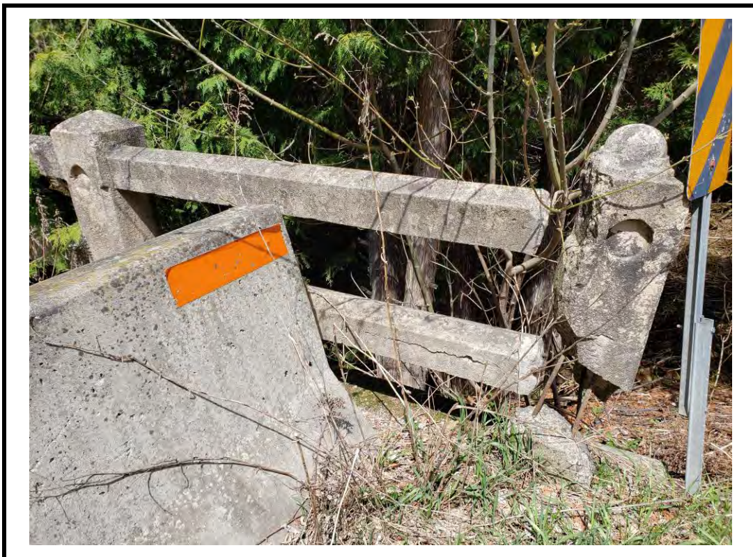
Photo 8 Full depth disintegration of concrete post in approach barrier system
