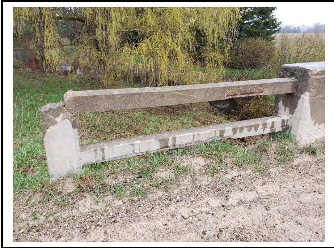
Photo 7 Spalls with exposed corroded reinforcement noted on approach barrier
