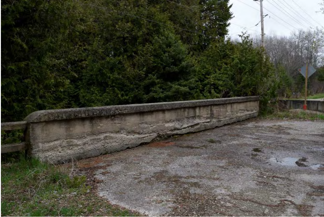
FIGURE 23: EAST SIDE OF BRIDGE 5-E SHOWING DEGRADATION OF CONCRETE
