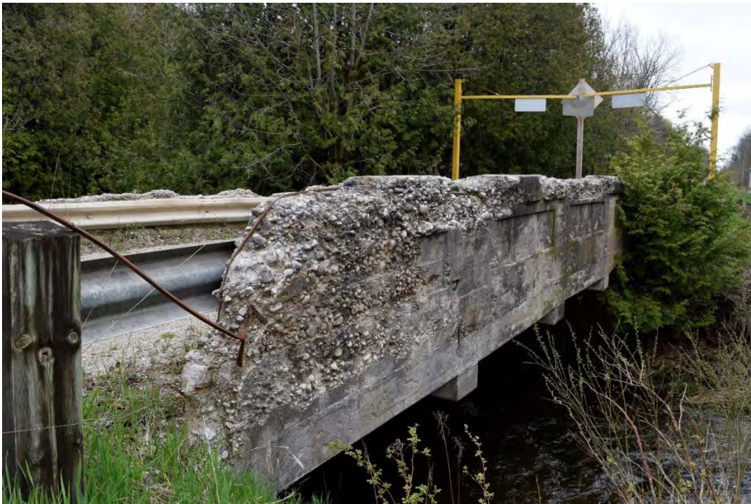
FIGURE 26: BRIDGE 7-E, DETERIORATED UPPER SUPPORT WALLS, WEST SIDE OF STRUCTURE
