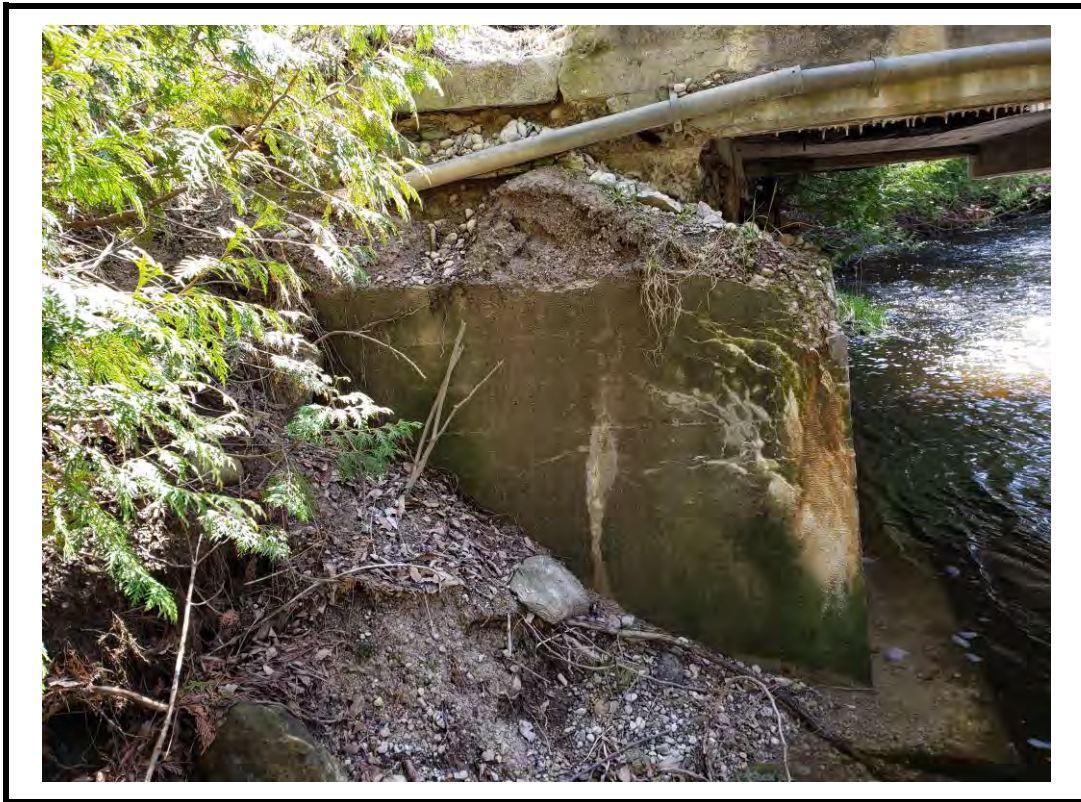
Photo 13 Spalls noted at south abutment and southeast wingwall interface.
