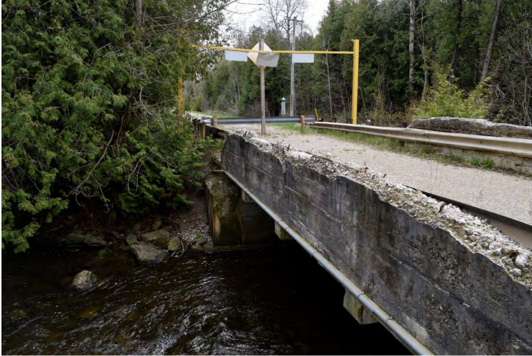
FIGURE 25: BRIDGE 7-E, DETERIORATED UPPER SUPPORT WALLS OF EAST SIDE OF STRUCTURE
