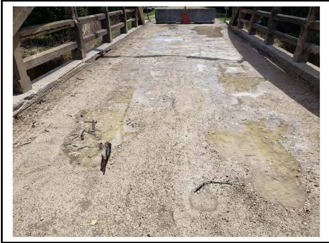
Photo 9 Spalls in exposed concrete deck top
