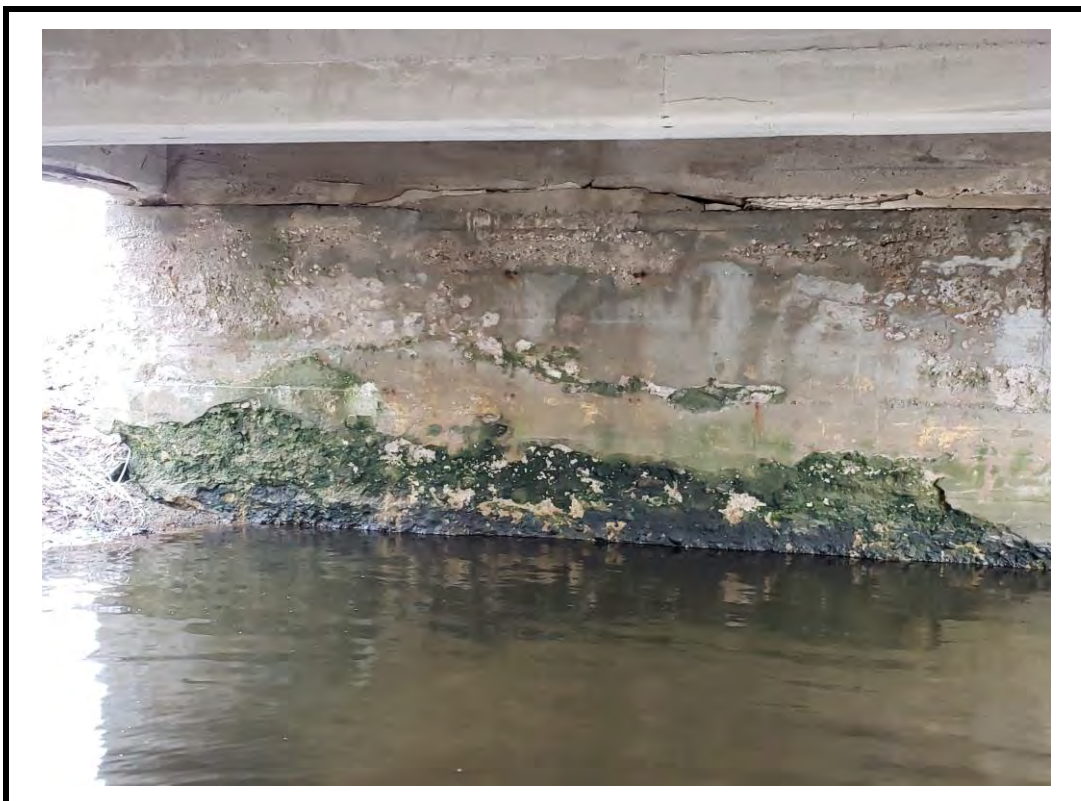
Photo 12 Sever scaling and erosion with horizontal cracks noted on north abutment wall
