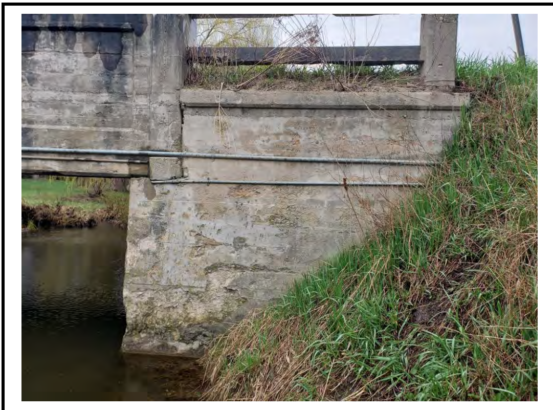
Photo 14 Concrete disintegration and spalls observed on wingwalls
