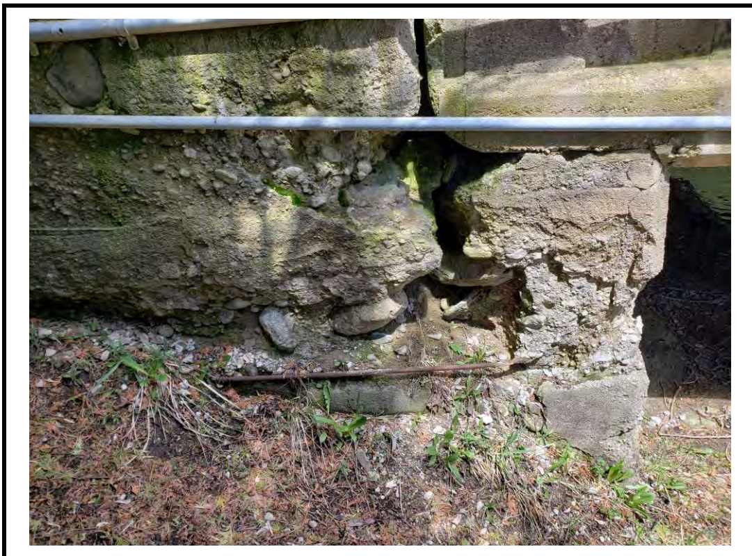
Photo 12 Severe concrete disintegration at NE wingwall
