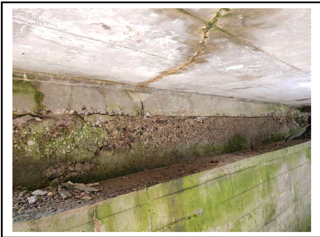
Photo 10 Medium cracks and map cracks with efflorescence
