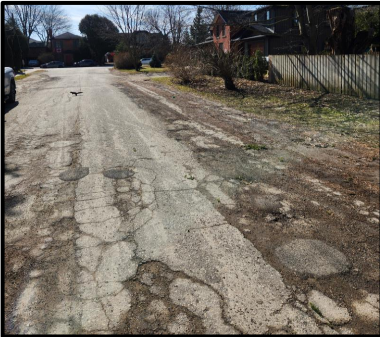
Smith Street Asphalt Condition (PCI 53-71 out of 100)
