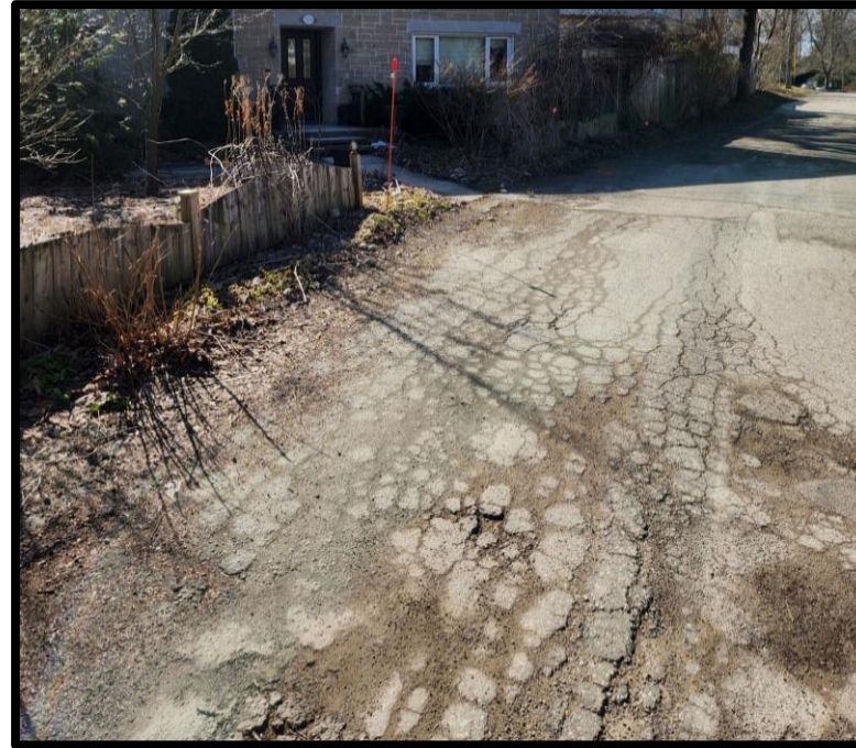
Victoria Crescent Asphalt Condition (PCI 51 out of 100)
