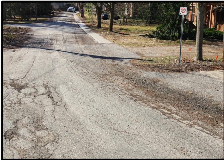
Victoria Crescent sidewalk termination
